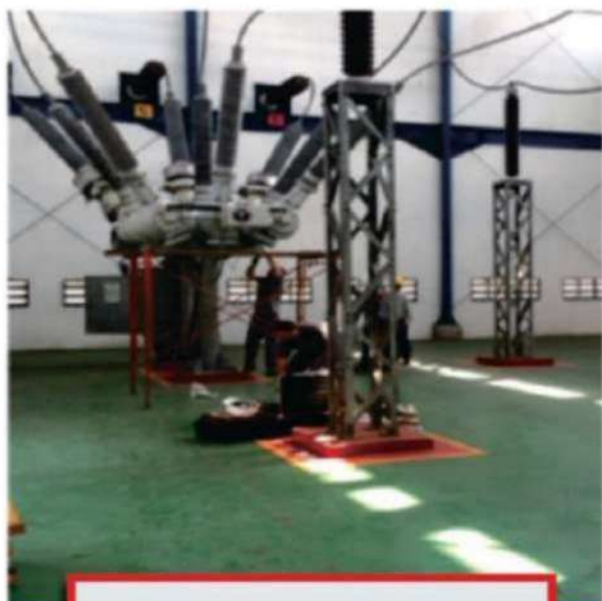
PT. JATIM TAMAN STEEL GI 150 kV 80 MVA
